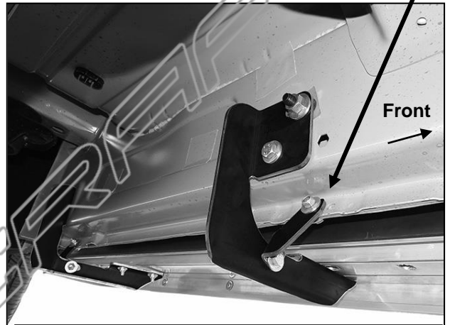
(Fig 14) Driver/left center and rear installation
