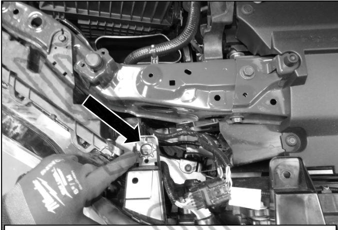
(Fig 2) With air intake out of the way, remove final bolt (arrow) attaching grille. (Passenger Side)
